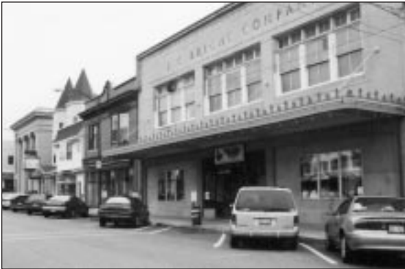
The former J.C. Bright Company Building retains its original decorative canopy held by iron rods.
