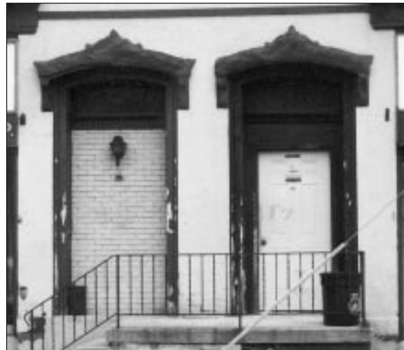
An inappropriate door renovation detracting from the building's historic appearance.
