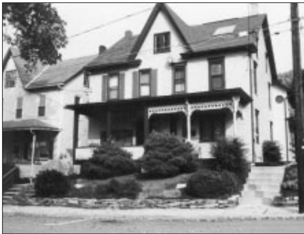
Original architectural detail has been removed on one-half of this double house.
